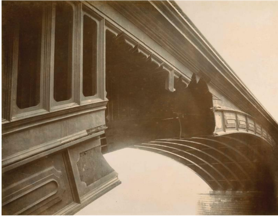
Photograph of Diamond damage; Rochester Bridge Trust.
